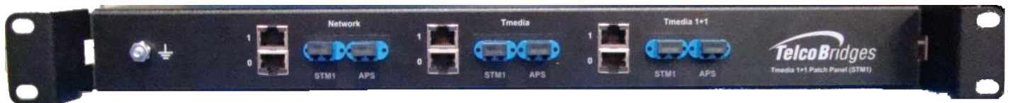
Tmedia TMG3200-STM1 1+1, Patch Panel (front view)
