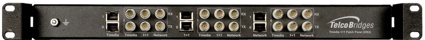
Tsig TSG3200-DS3 1+1, Patch Panel (front view)
